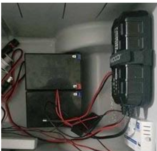
Fig. 3.1: 12V 16Ah Batteries
